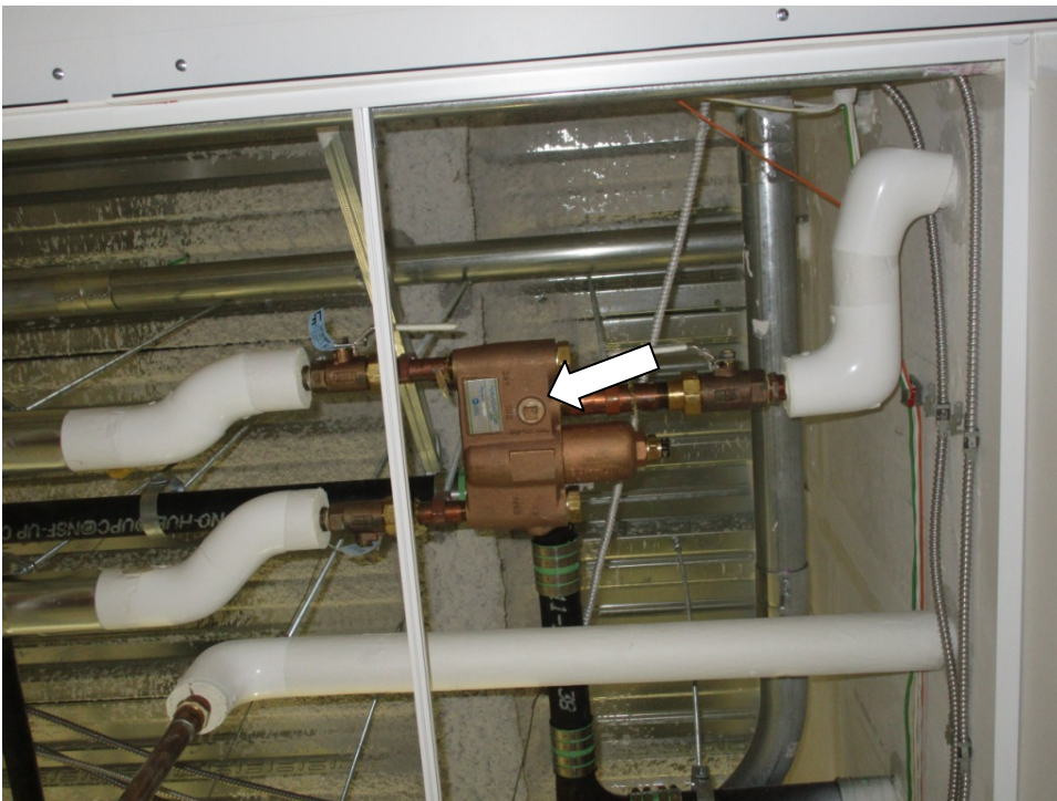
Photo 3-10 Biology Prep Room East 386 – Missing thermometer gauge on TMV
