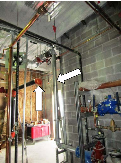
Photo 04 Level 01 – Domestic water service and fire service piping split.
