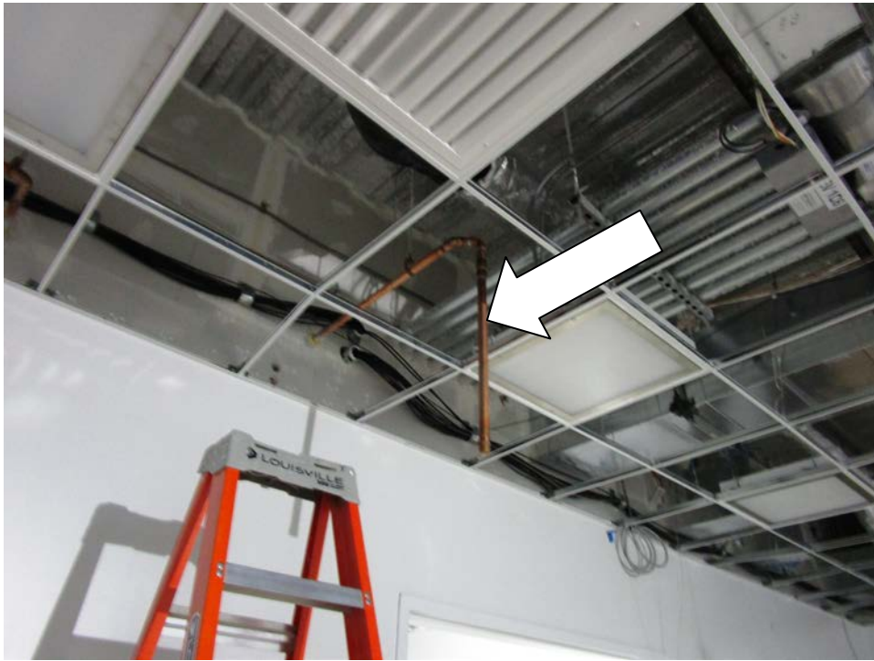
Photo 1-3 Cadaver Lab 191 – Emergency shower discharge piping not insulated.
