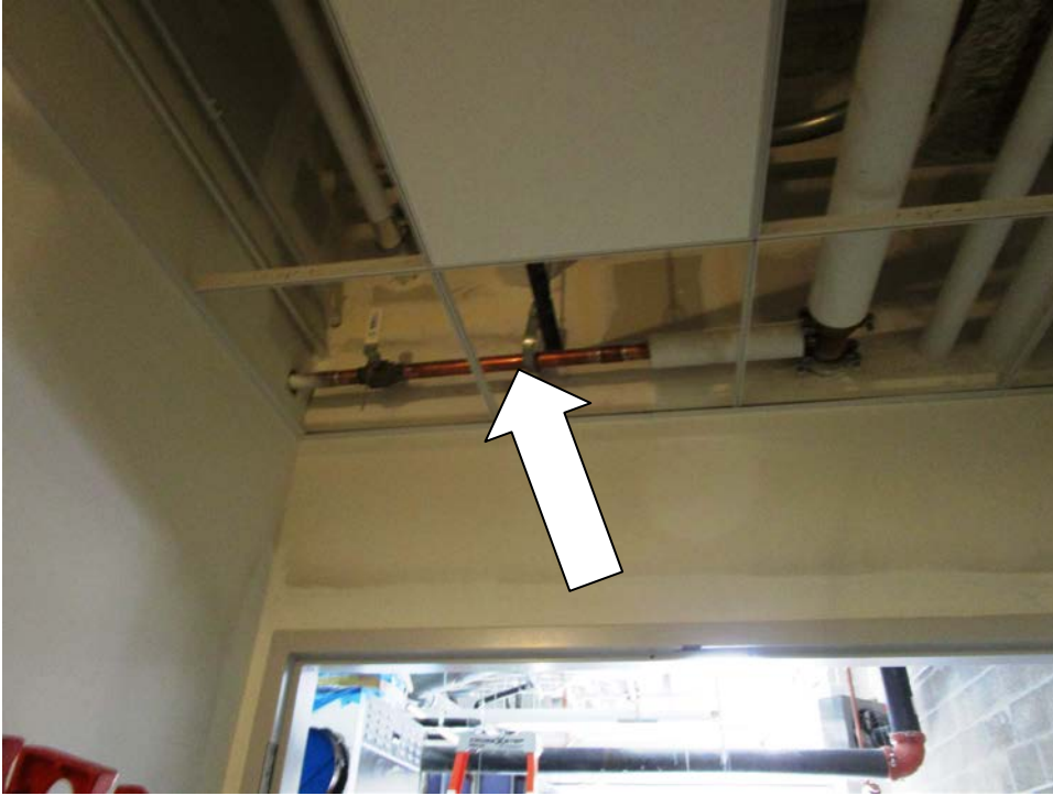
Photo 1-1 Corridor C180 (outside Mechanical Room 178) – Piping not insulated.
