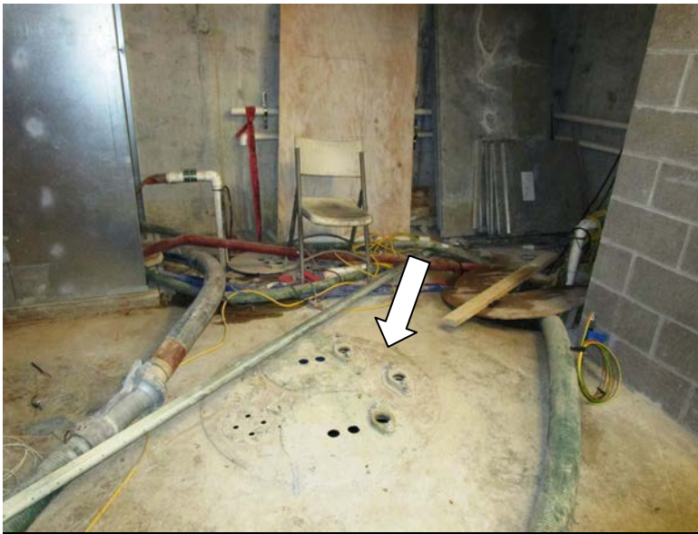
Photo 01 Level 0 – Sump pumps not yet installed.
