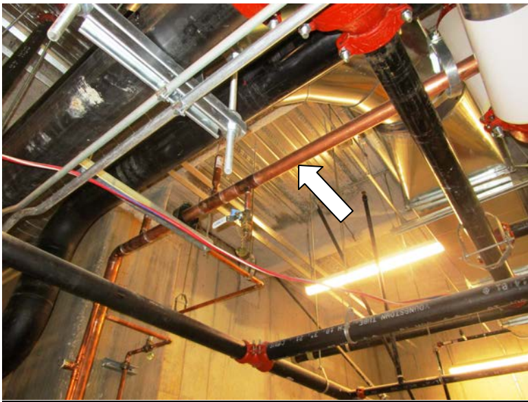
Photo 02 Level 0 – Domestic water piping not yet insulated.
