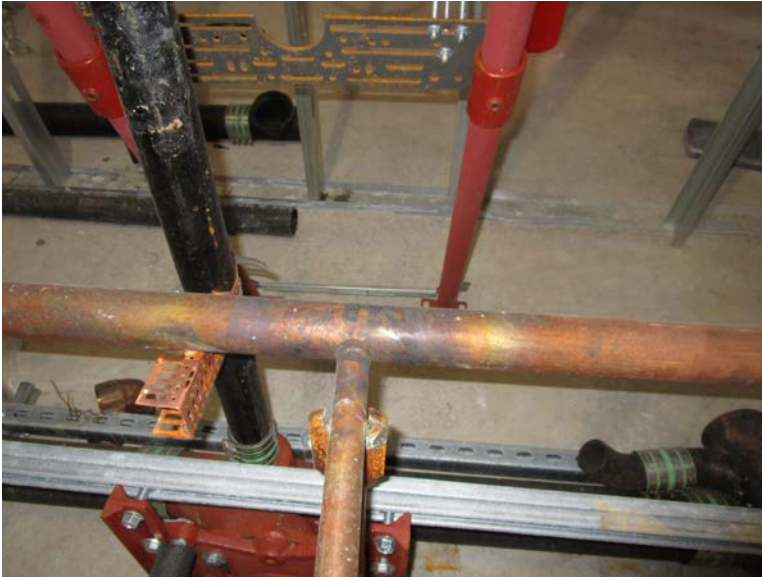
Photo 1 Brazed pipe tap
