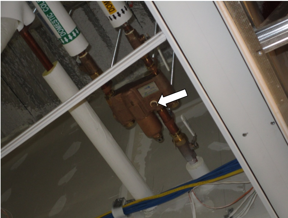
Photo 3-7 Biology Research Lab (Neurobiology) 374A – Missing thermometer gauge on TMV
