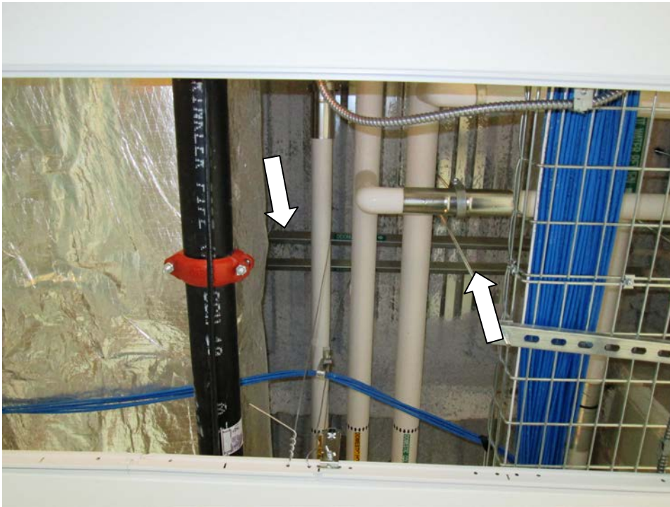
Photo 2-1 Corridor C280 – Di / RO piping not wrapped where crossing in corridor.
