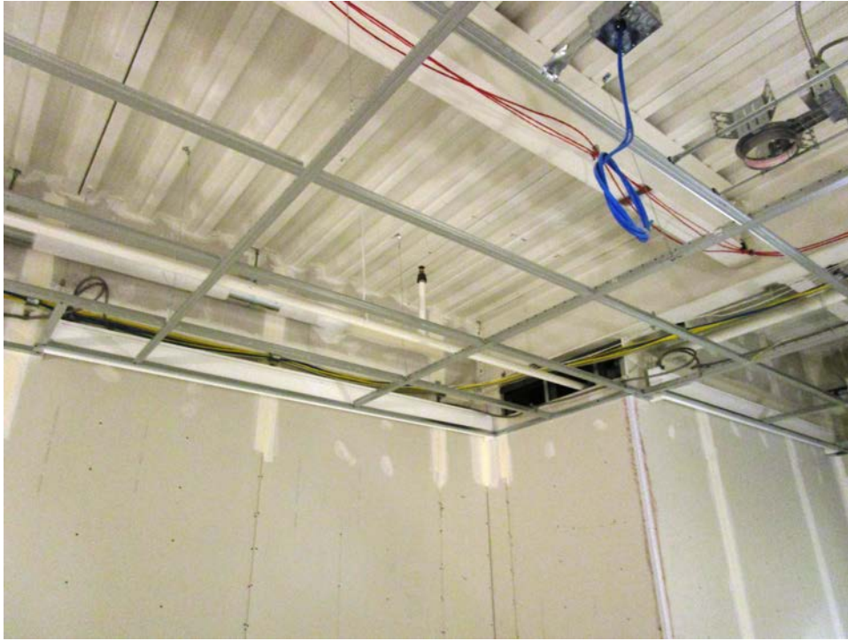
Photo 1-7 EAB Connector – New sprinkler work not completed.
