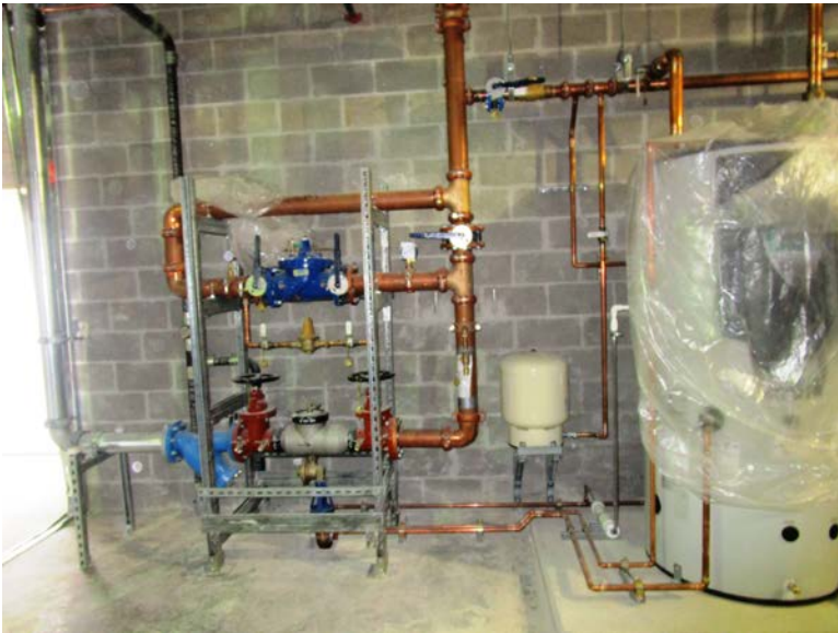
Photo 06 Level 01 – Domestic water service backflow preventer and PRV station.
