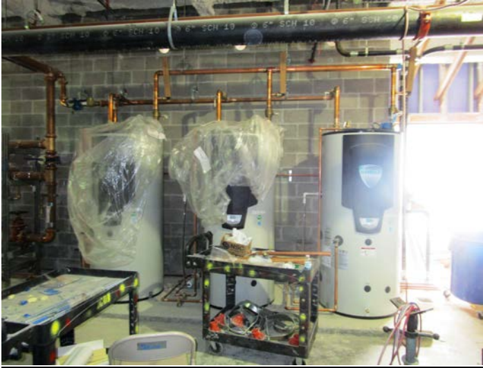
Photo 05 Level 01 – Domestic hot water heaters, installed and piped.
