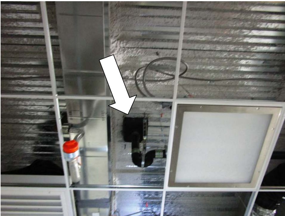
Photo 1-2 Cadaver Lab 191 – Floor sink supported by single underfloor brace.
