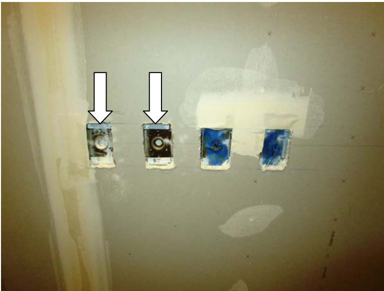
Photo 10 Level 01 Sim Lab - Med Gas wall inlets and outlets to be cleaned and covered to protect from dust.
