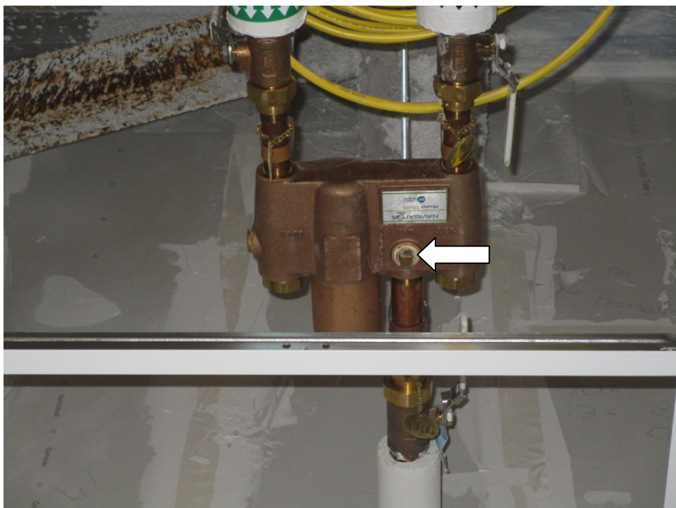
Photo 3-4 Biology Autoclave Room 372B – Missing thermometer gauge on TMV
