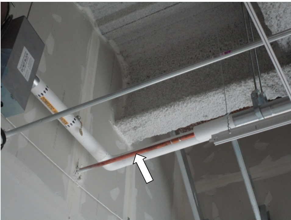
Photo 3-8 Biology Research Lab (Neurobiology) 374A – Missing pipe insulation
